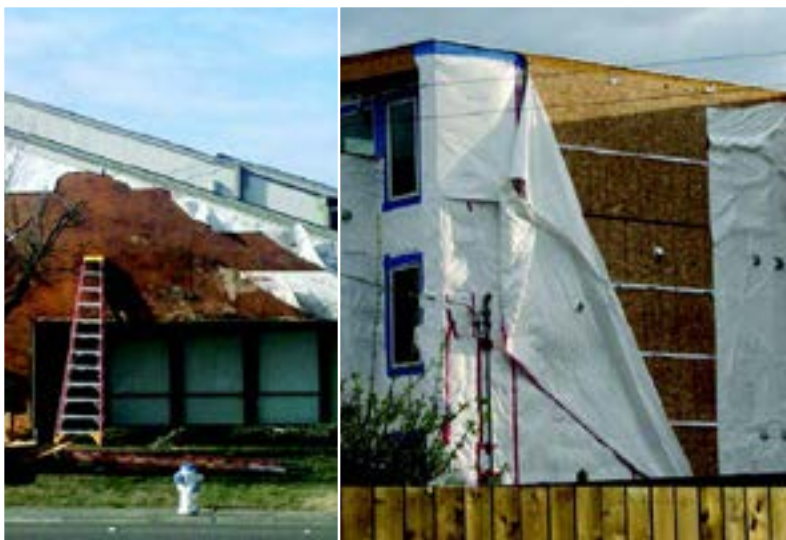
Does this problem look familiar? Avoid it by using Backstop NTX and AquaFlash by Dryvit!
